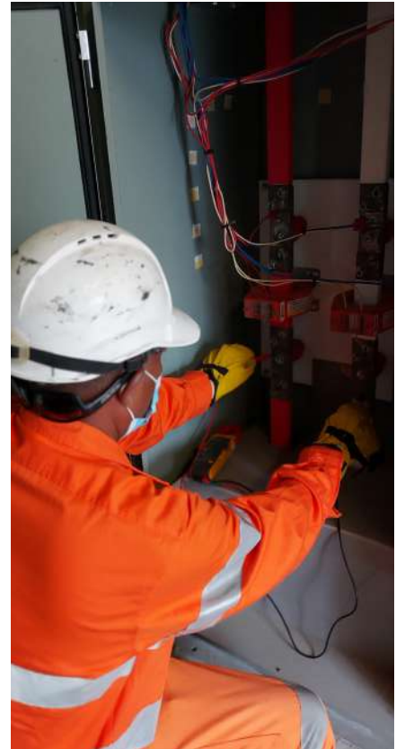
David Siriu (Principal Electrical Inspector) carrying out customer main switch board verification.
