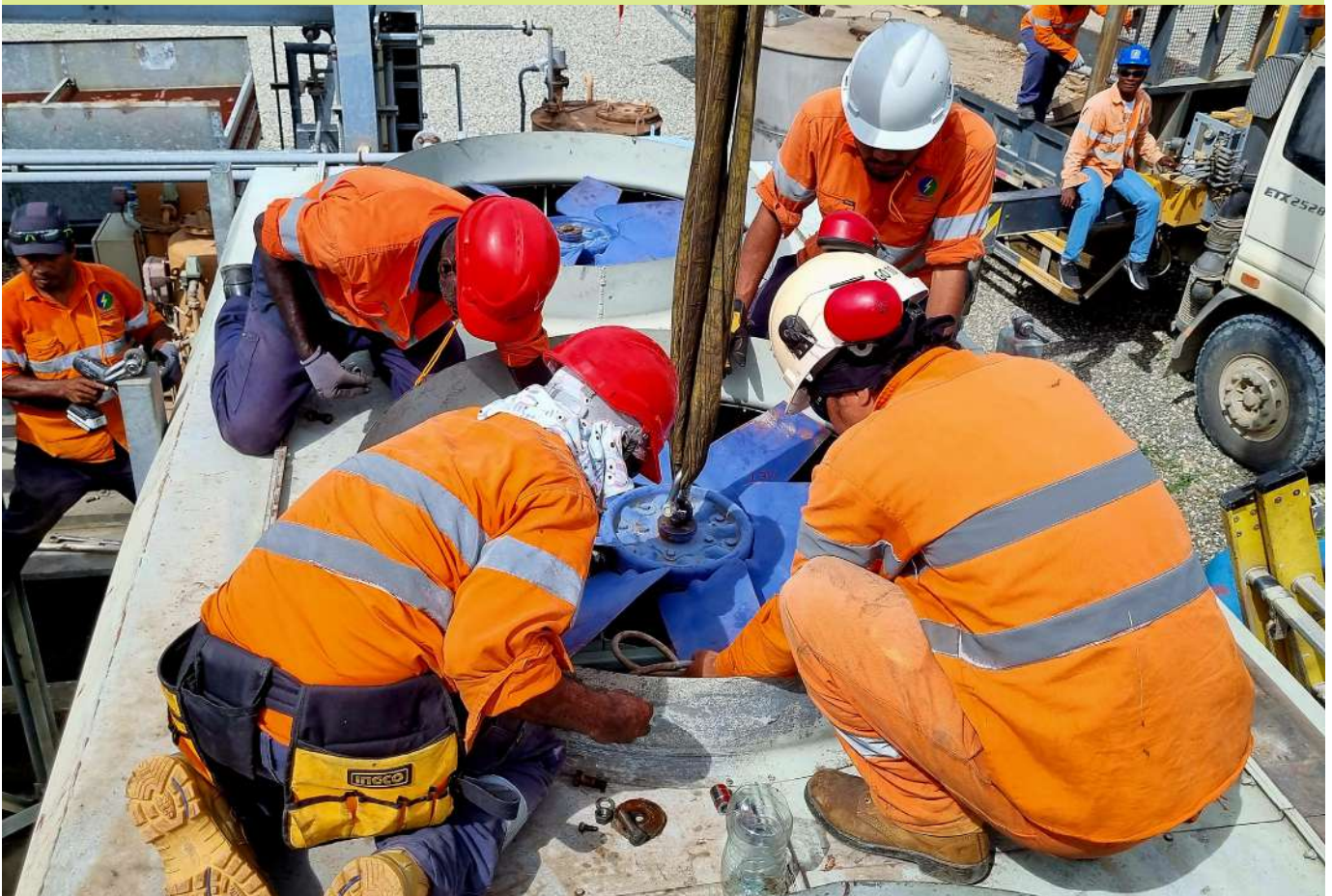
Lungga Electrical Team
